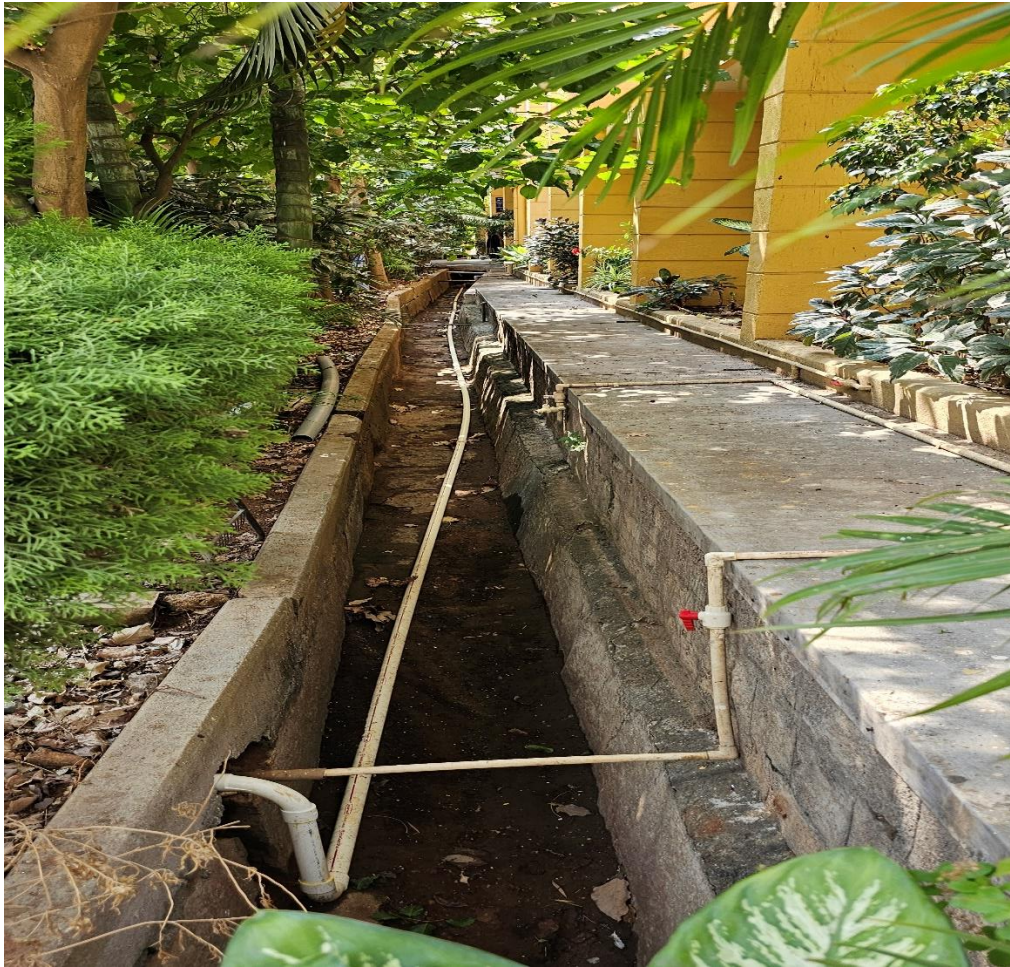
Open Rain water channels
