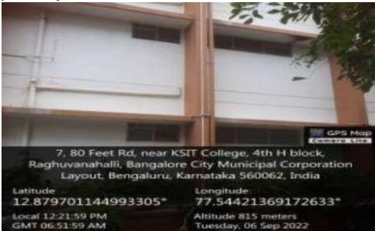
Rain water pipes
