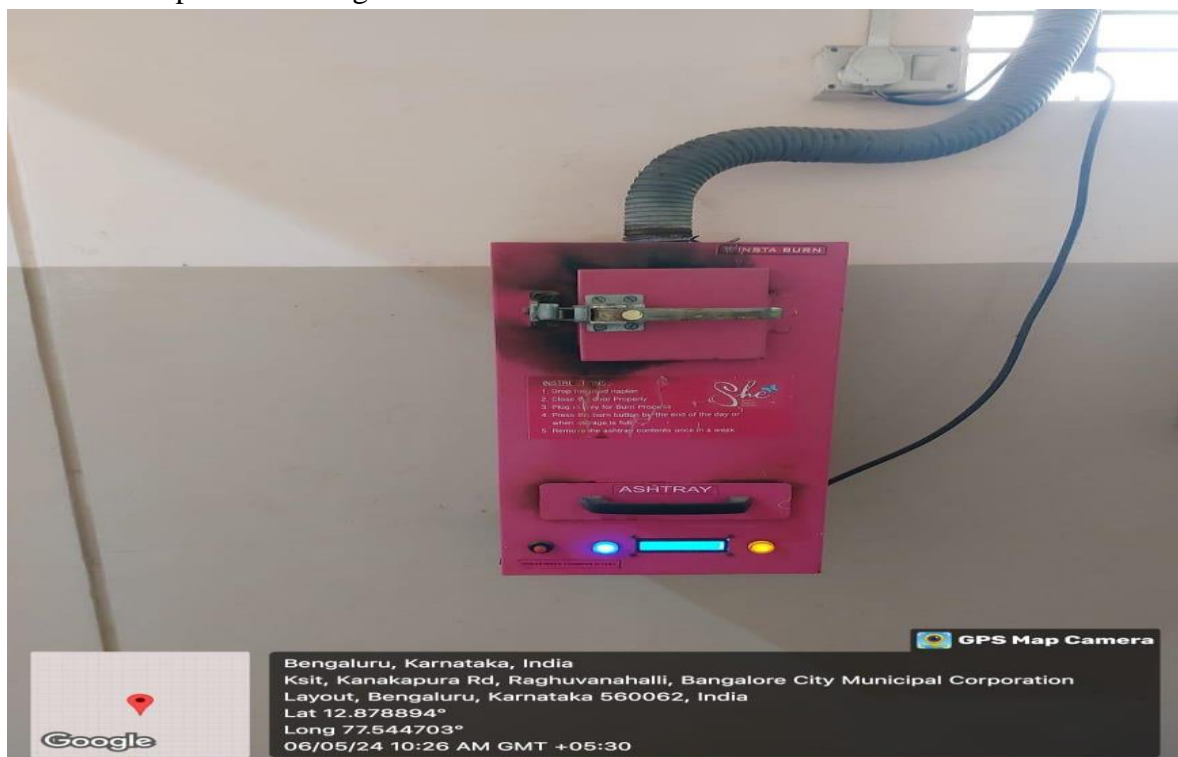
Sanitary pad Incinerator
