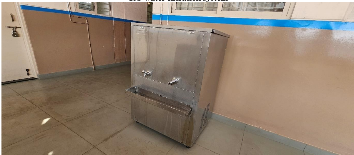
RO water dispenser
