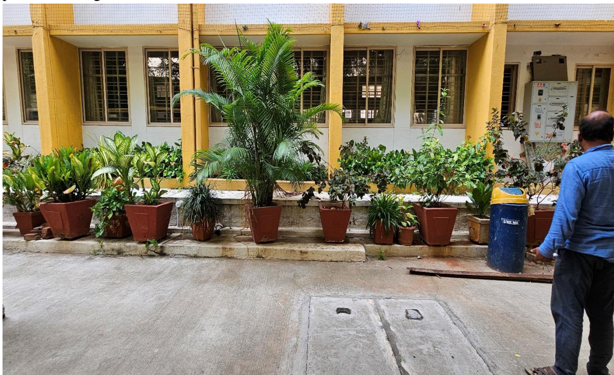
Rain water pipes and recharge pits
