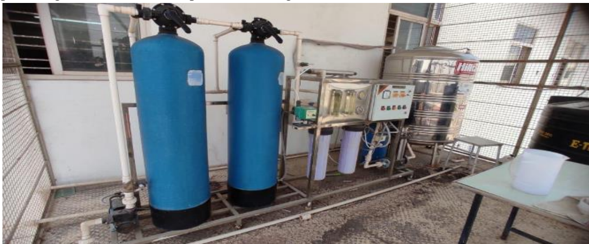
RO water filtration system
