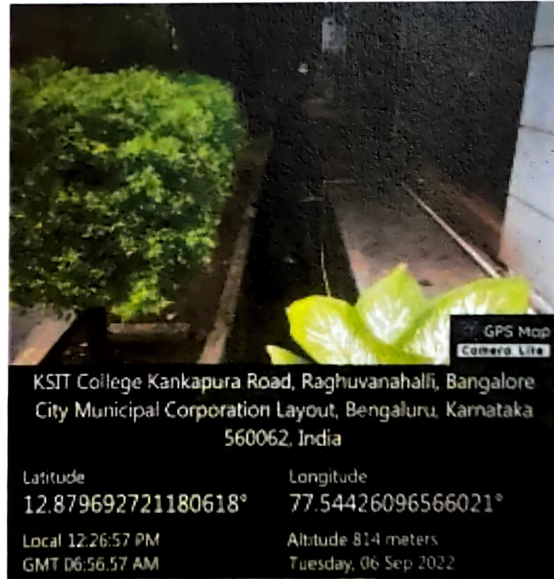
Roof top rain water harvesting recharge pit
